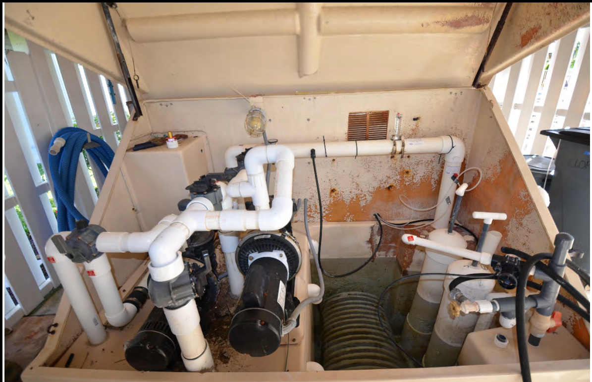
VIEW OF TYPICAL POOL EQUIPMENT
