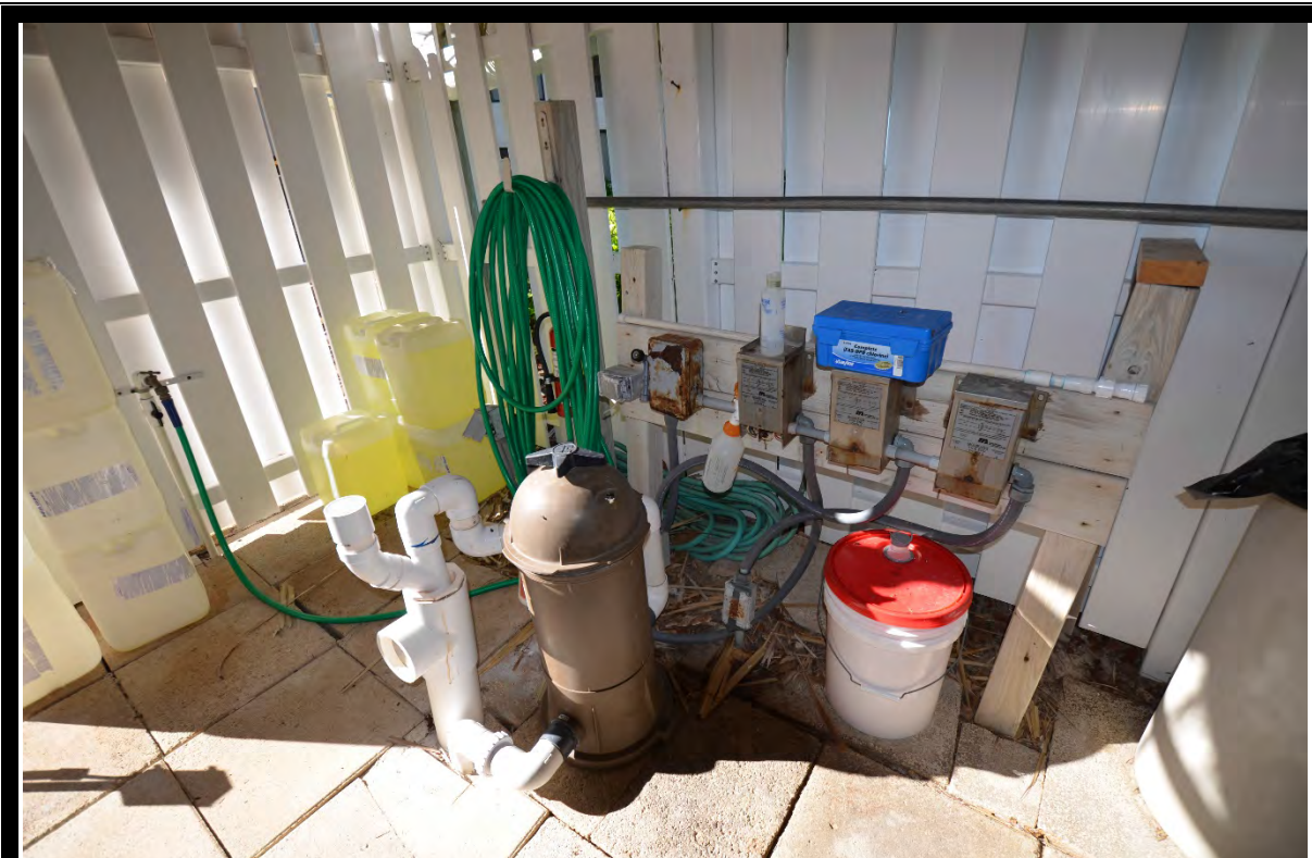
VIEW OF TYPICAL POOL EQUIPMENT
