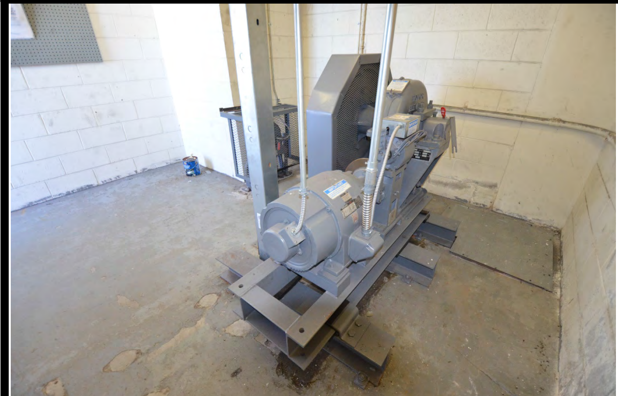
VIEW OF TYPICAL BUILDING MECHANICAL EQUIPMENT
