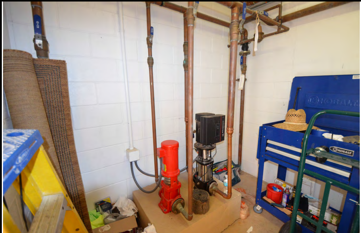
VIEW OF TYPICAL BUILDING MECHANICAL EQUIPMENT
