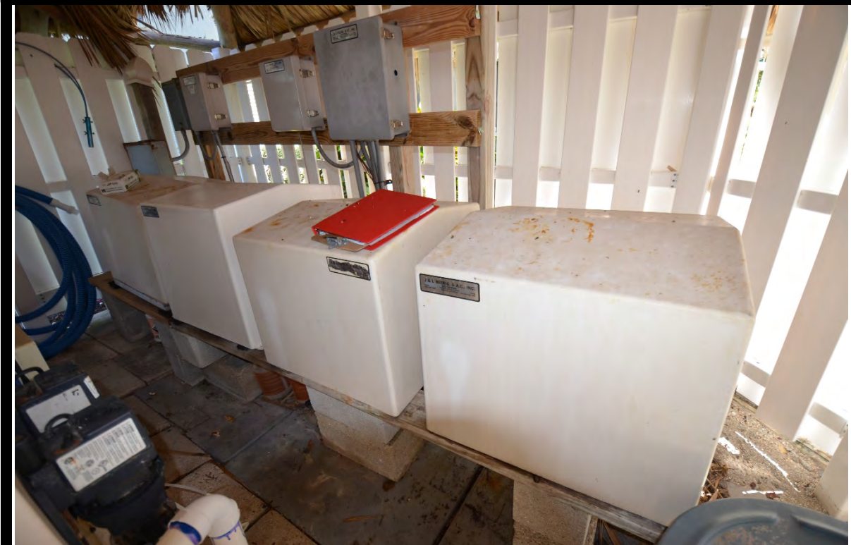
VIEW OF TYPICAL POOL EQUIPMENT
