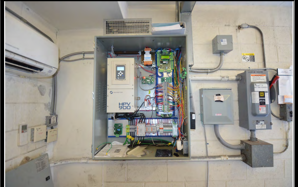
VIEW OF TYPICAL BUILDING MECHANICAL EQUIPMENT
