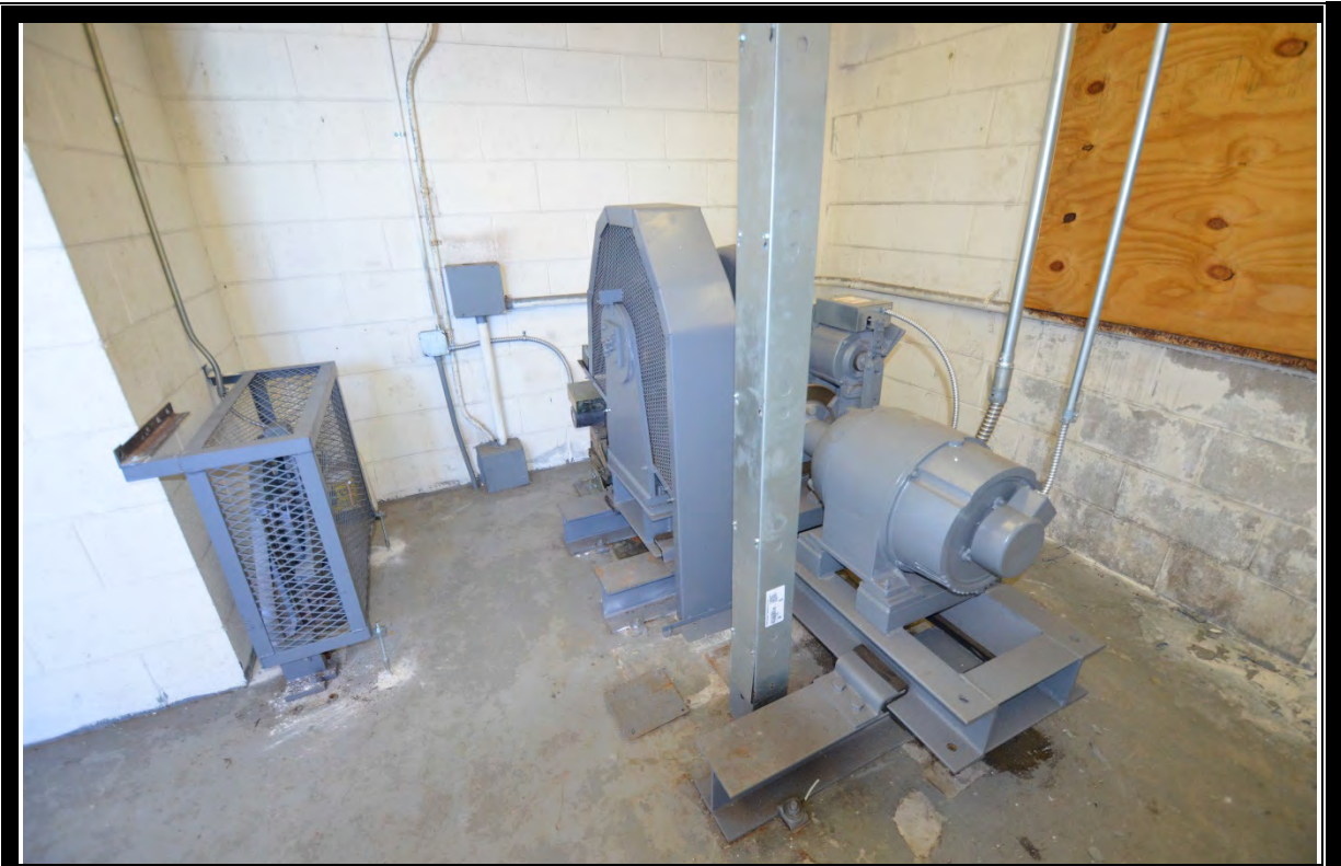
VIEW OF TYPICAL BUILDING MECHANICAL EQUIPMENT
