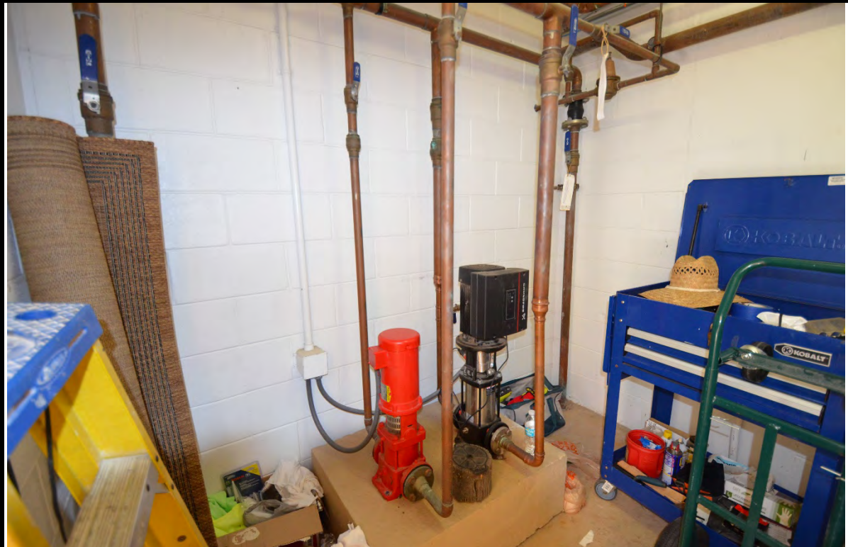
VIEW OF TYPICAL BUILDING MECHANICAL EQUIPMENT
