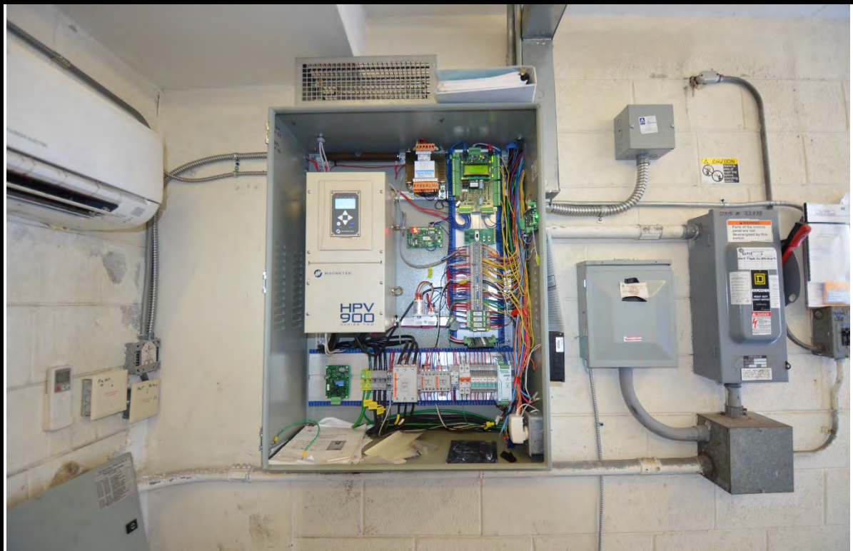
VIEW OF TYPICAL BUILDING MECHANICAL EQUIPMENT
