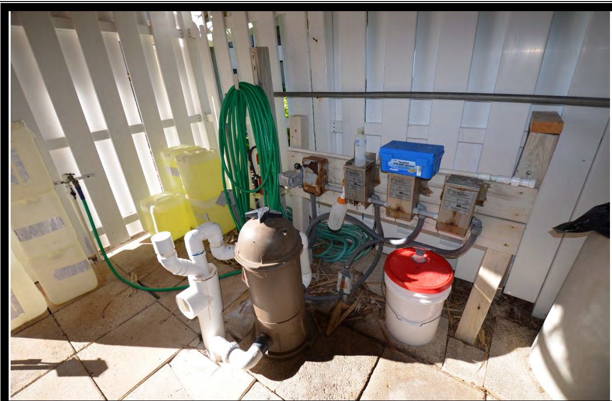
VIEW OF TYPICAL POOL EQUIPMENT
