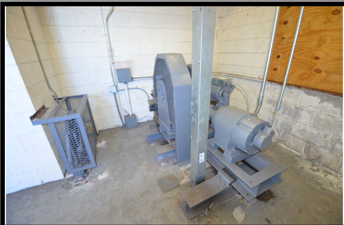
VIEW OF TYPICAL BUILDING MECHANICAL EQUIPMENT
