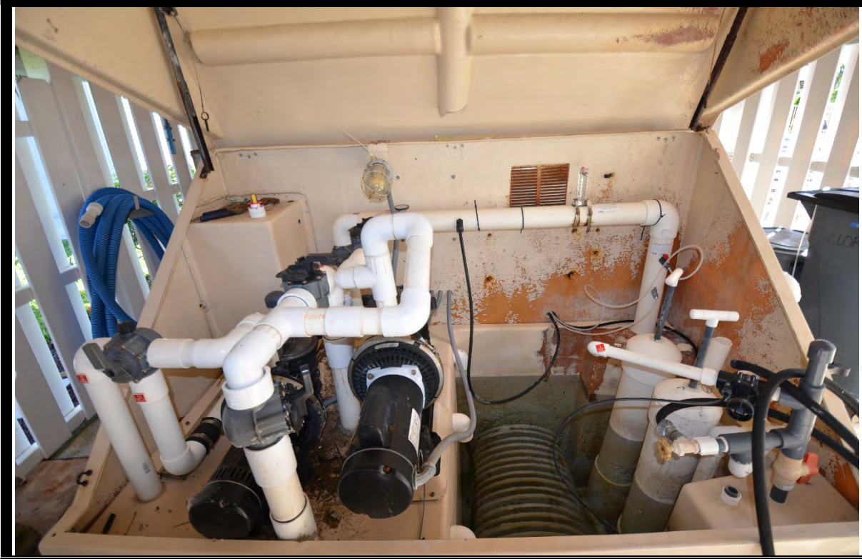
VIEW OF TYPICAL POOL EQUIPMENT
