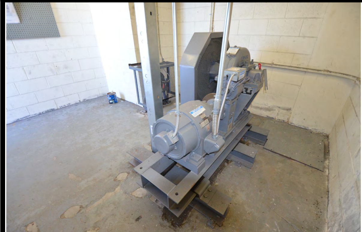
VIEW OF TYPICAL BUILDING MECHANICAL EQUIPMENT
