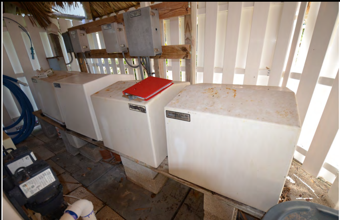
VIEW OF TYPICAL POOL EQUIPMENT
