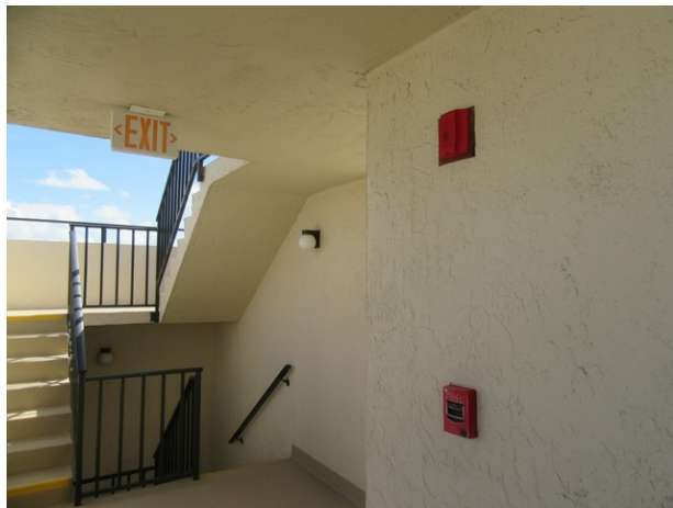
Life safety system components
