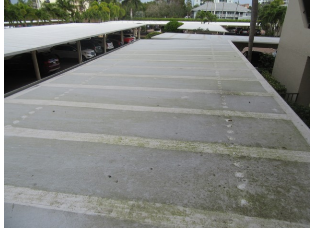
Carport thermoplastic roof
