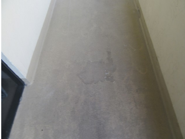
Waterproof coating deterioration
