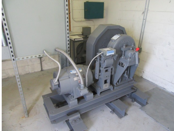
Elevator machine and hoist
