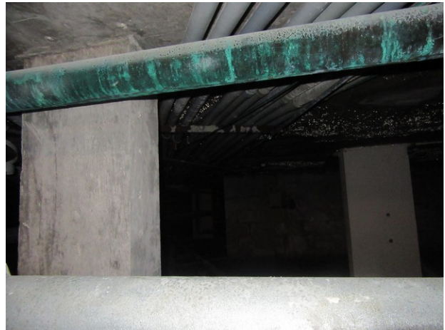
Domestic water pipe
