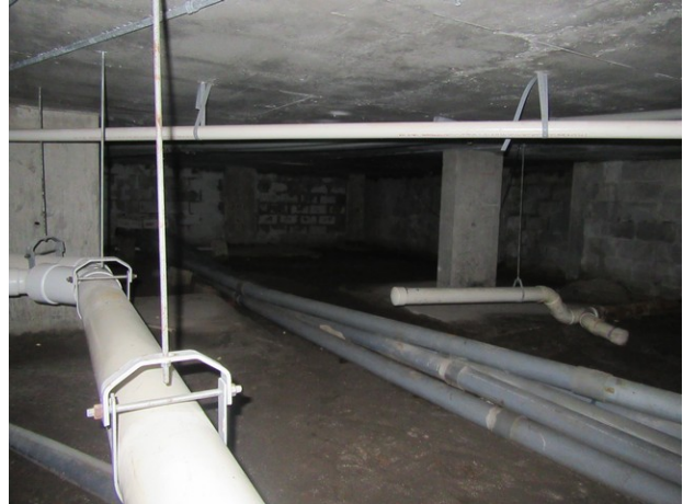
Sanitary waste pipes (Replaced in 2010)
