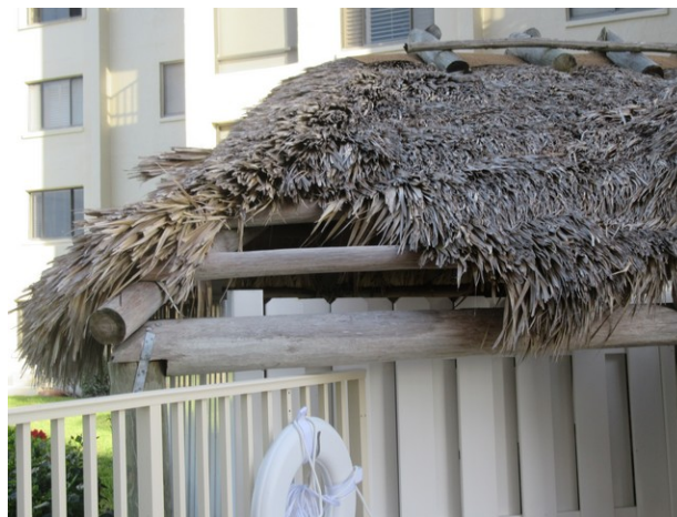
Missing thatched roof
