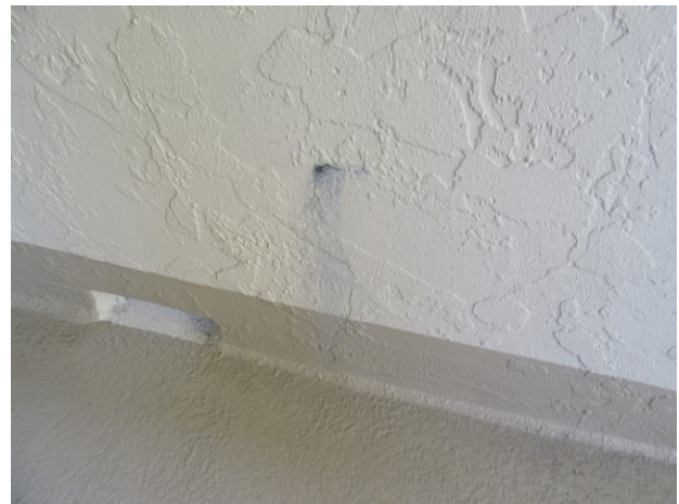
Isolated paint finish deterioration
