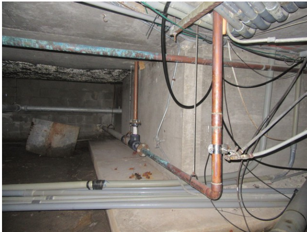
Domestic water pipes
