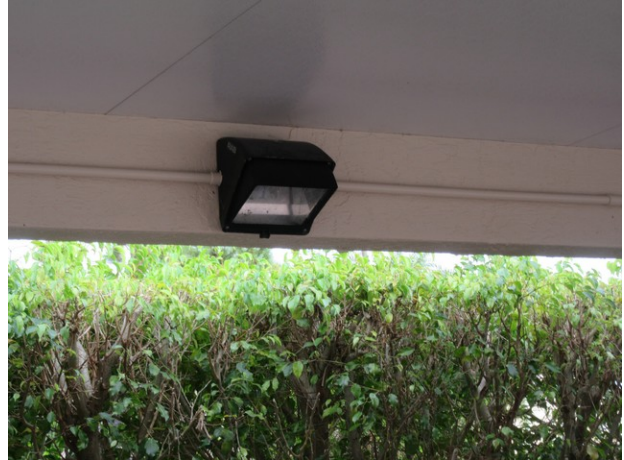
Carport light fixture
