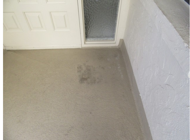
Waterproof coating deterioration
