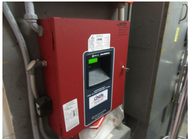
Life safety system control panel
