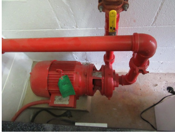
Fire suppression system pump
