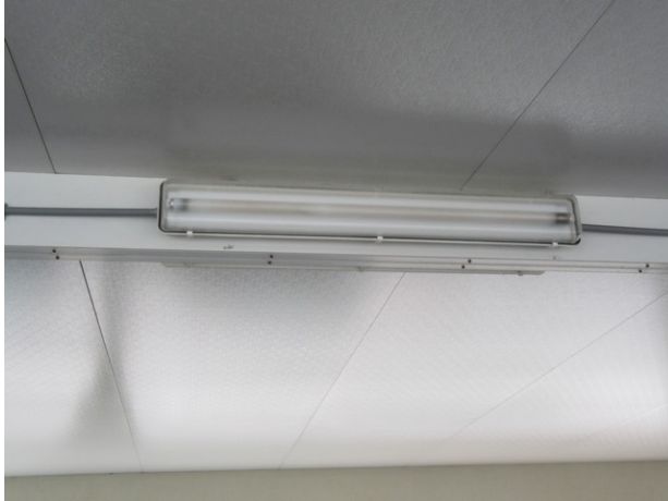
Carport light fixture
