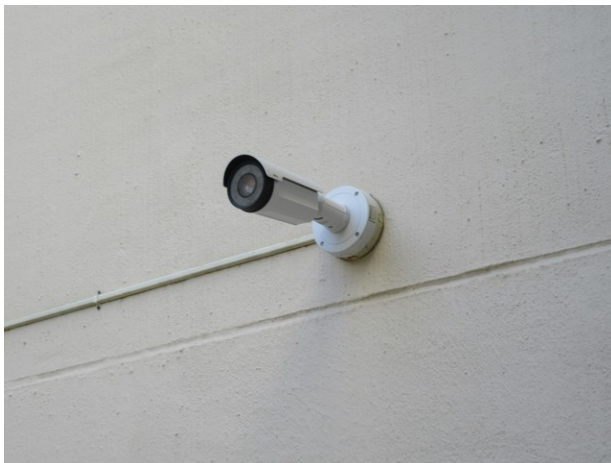
Security system camera
