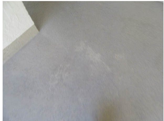
Waterproof coating deterioration
