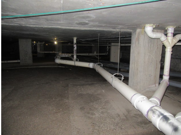
Sanitary waste pipes (Replaced in 2010)
